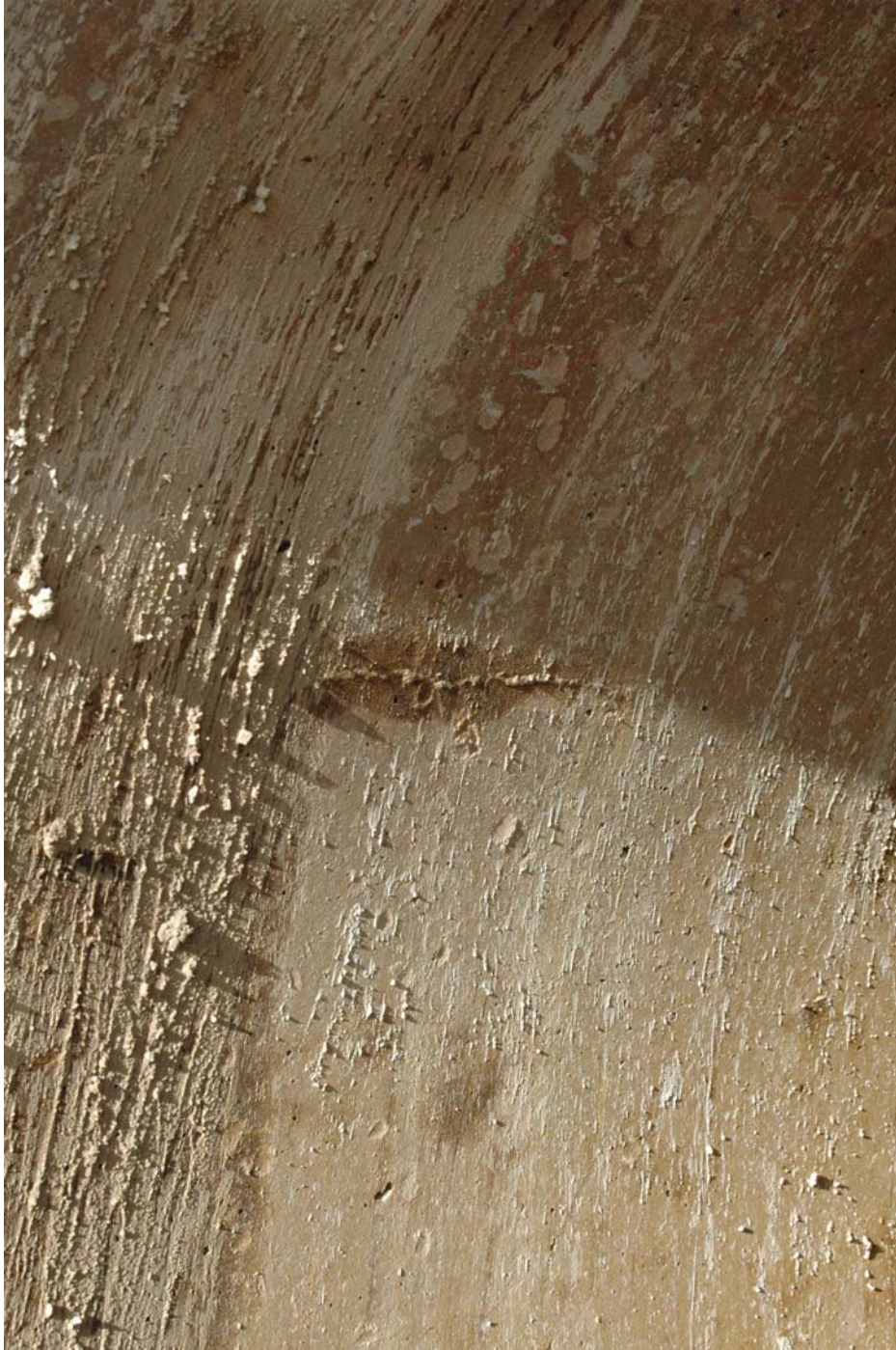
Crack on interior of the pipe at the location of the wire break damage, along springline. Other cracks in the pipe could not be observed due to the presence of debris and silt in the pipe.
