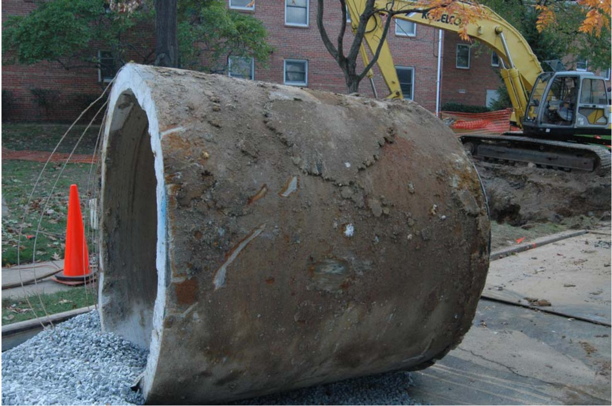
Spigot Portion of the pipe. No damage was observed on this portion of the pipe.
