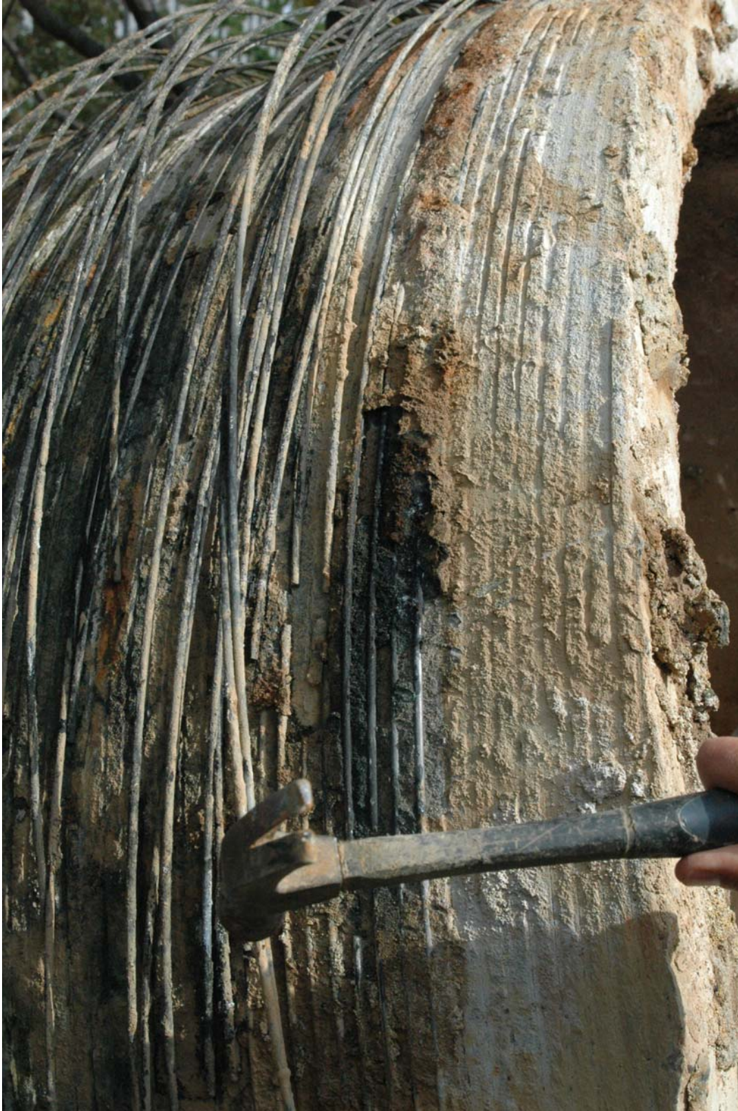
Close up of some of the wire break damage. The wires had a black film on them. Significant quantities of rust were not observed.
