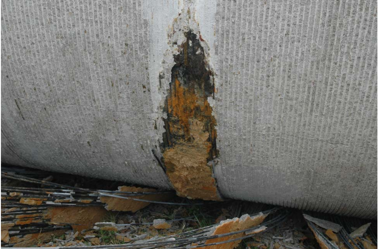
Corrosion product on concrete core at the location of wire break zone 1.
