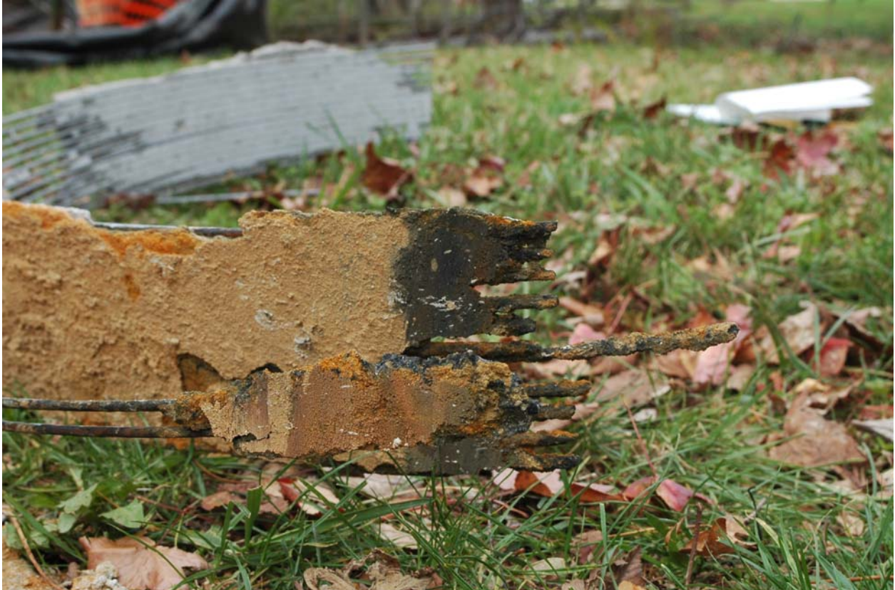
Group of wire breaks that were removed from wire break zone 1. Photo shows 12 wire breaks (some wires are not clearly visible). There was a total of 16 wire breaks in this zone.
