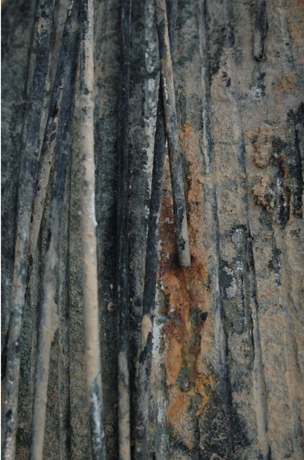
Close up of wire breaks.
