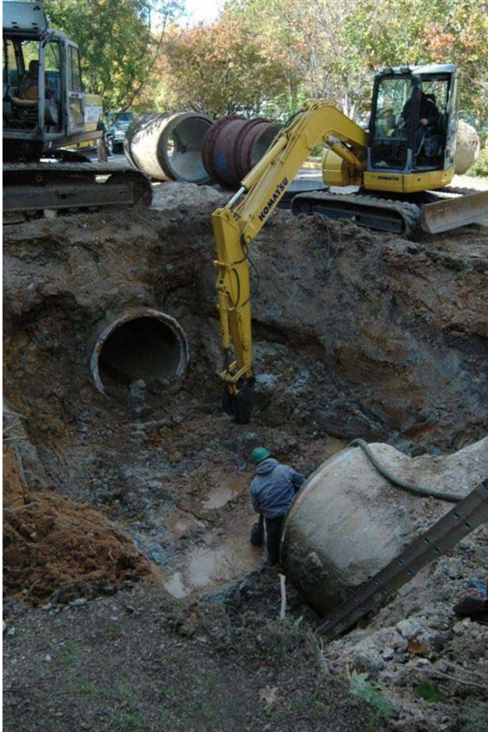
Photograph of the excavation. The pipe at the top of the photo is G295. It was confirmed that G295 was next to an air release valve, which is consistent with the inspection records. Thus the correct pipe was excavated.
