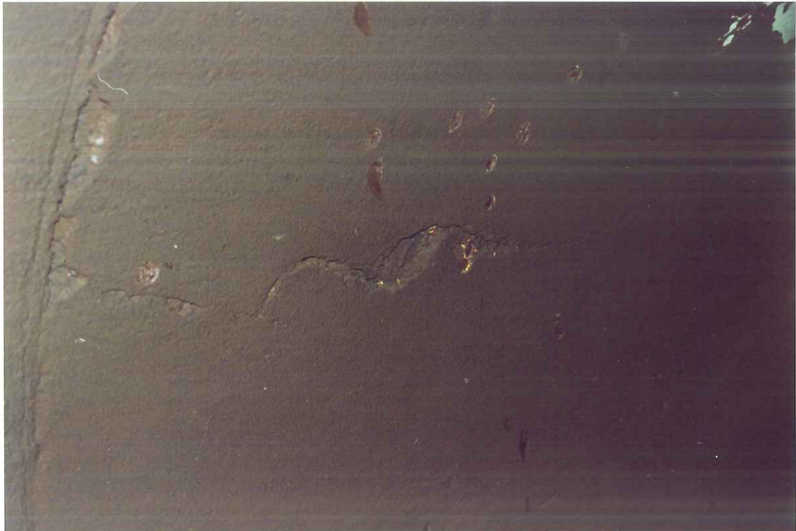
Figure 1. Cracked lining on the west side of the 2 meter by 1.5 meter reducer by valve #7, K0-260.
