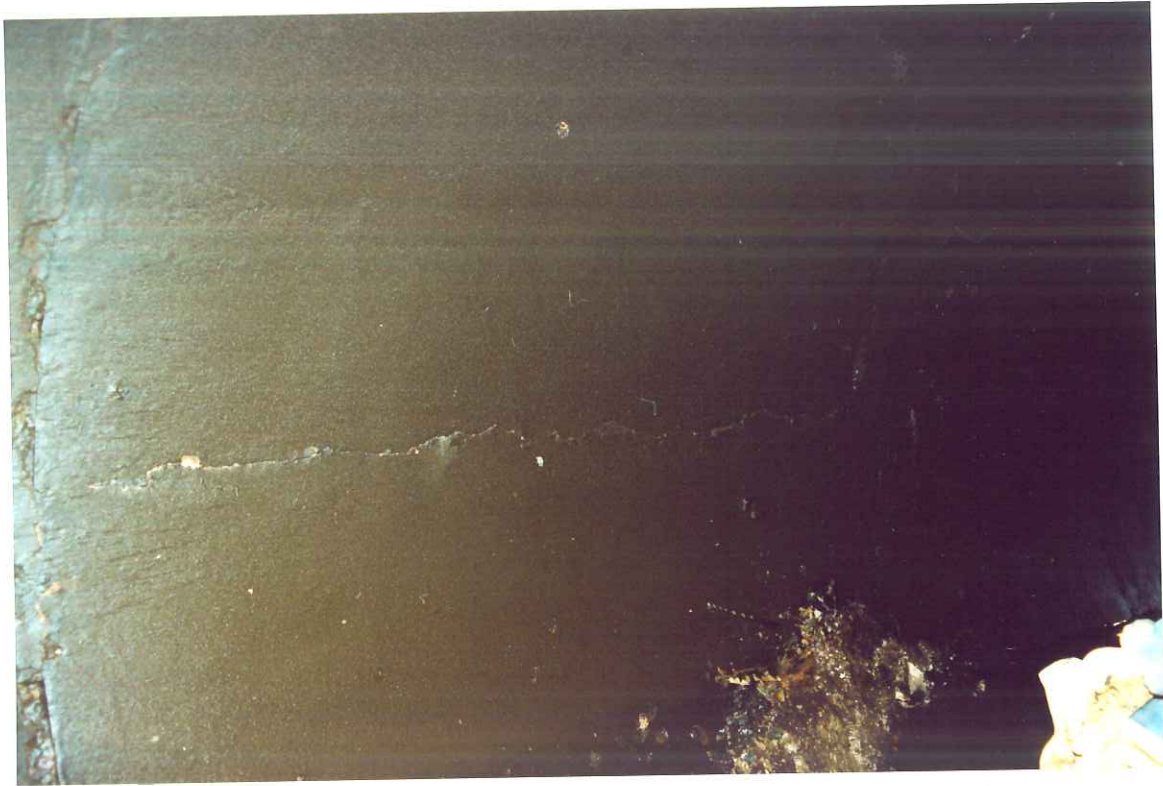
Figure 13. Cracked and hollow lining on the east side of the northern steel short at the failure location 43 to 44 joints south of the entry port at K3+856.
