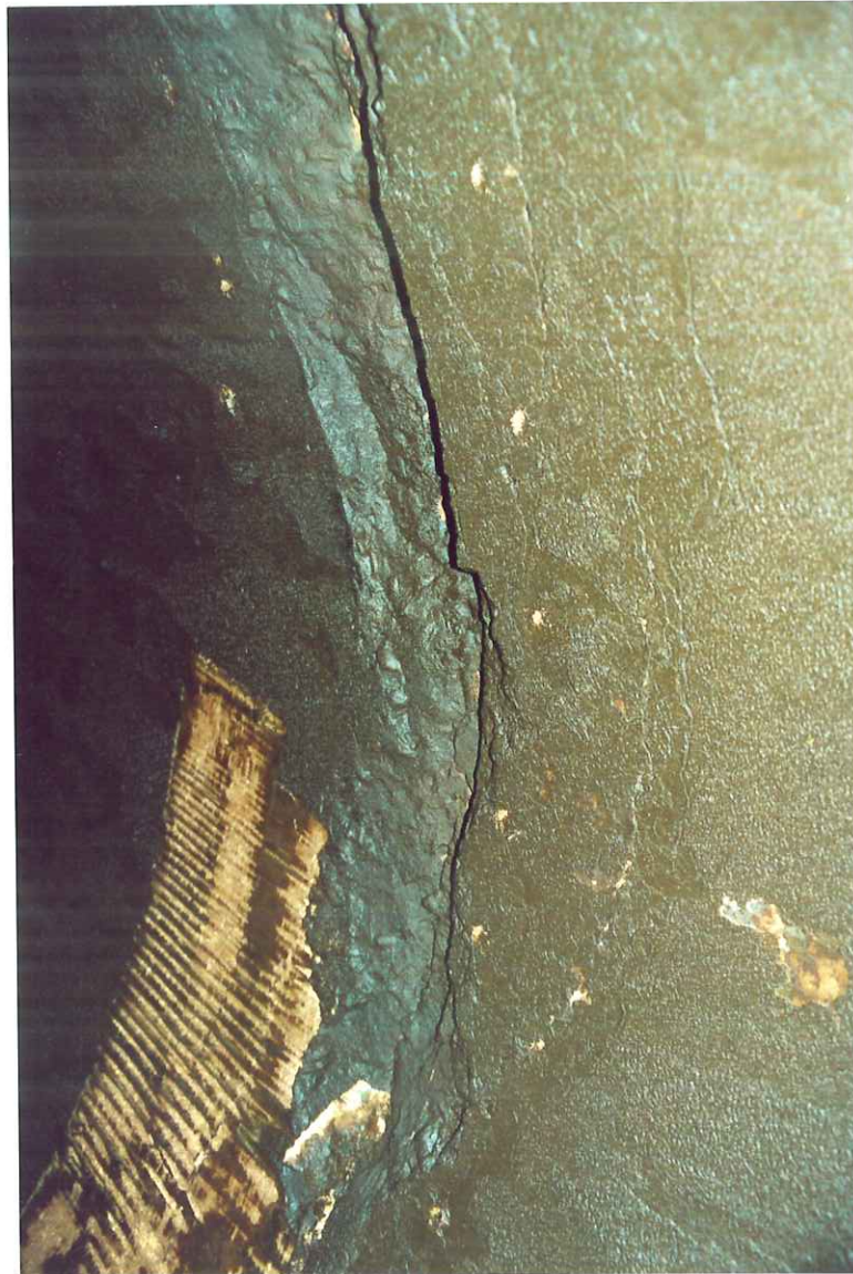
Figure 7. Spalled joint above the west springline of the 25 th joint north of the blow-off at K0+794±.
