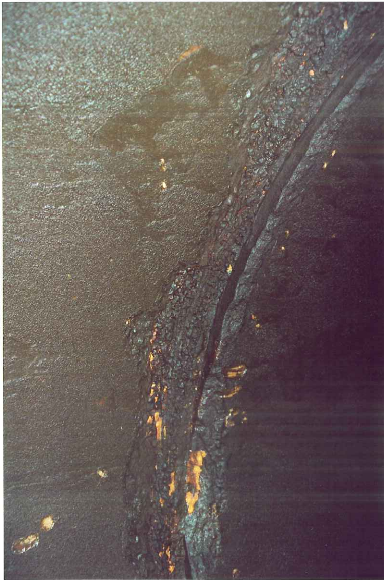
Figure 4. Spalled joint above the east springline of the 14 th joint north of the entry port at K0+539.
