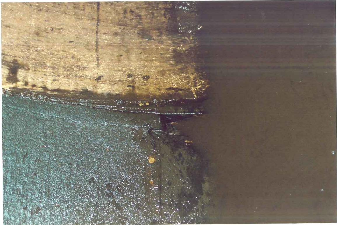
Figure 8. Joint mortar missing at the invert of the 15 th joint north of the entry port at K1+291.
