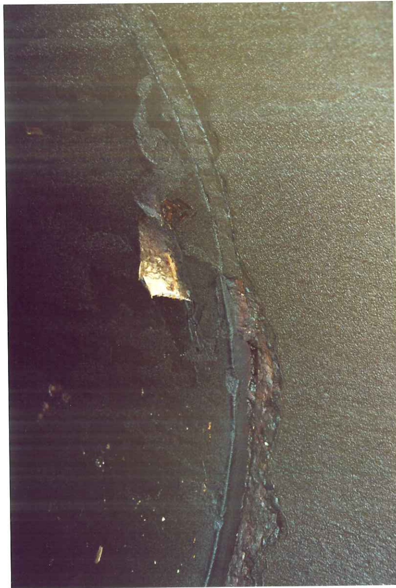
Figure 11. Spalled joint mortar and lining patch below the west springline at the north joint of the steel special with entry port at K2+952.
