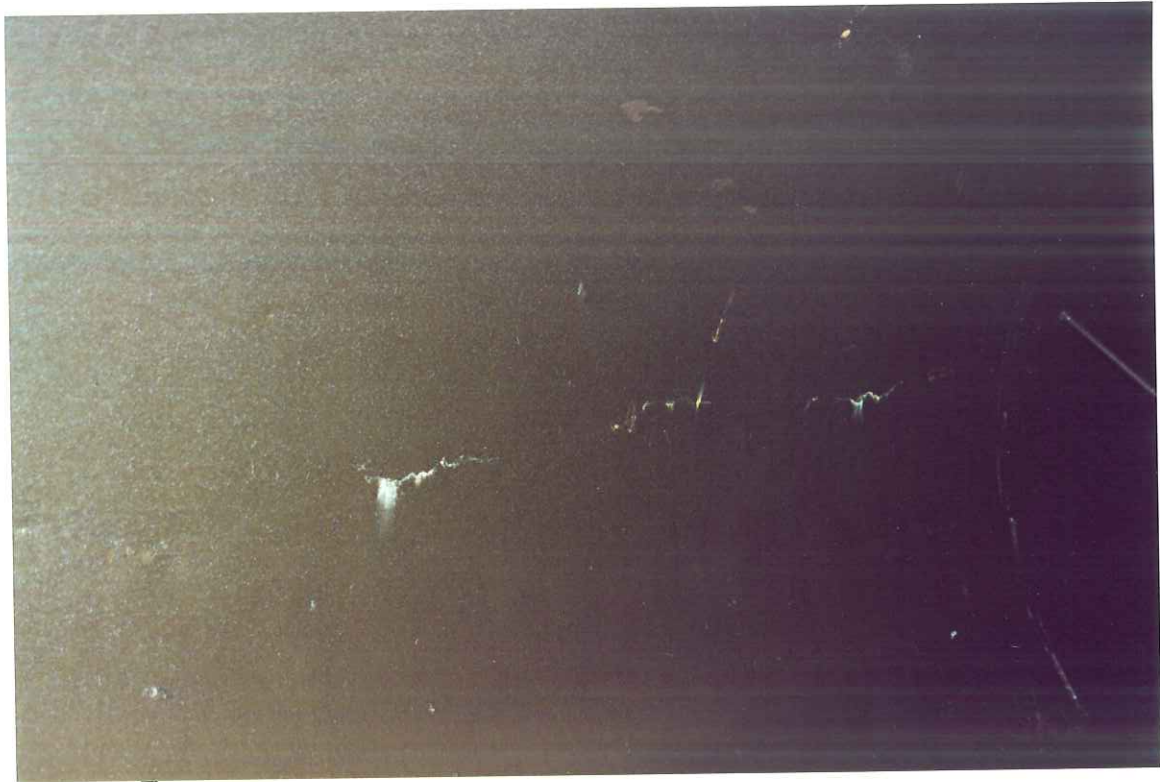
Figure 15. Cracked and hollow lining on the east side of the southern steel short at the failure location 43 to 44 joints south of the entry port at K3+856.
