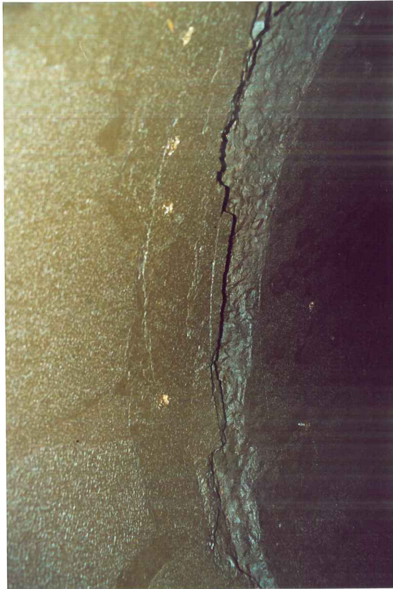
Figure 6. Spalled joint above the east springline of the 25 th joint north of the blow-off at K0+794±.
