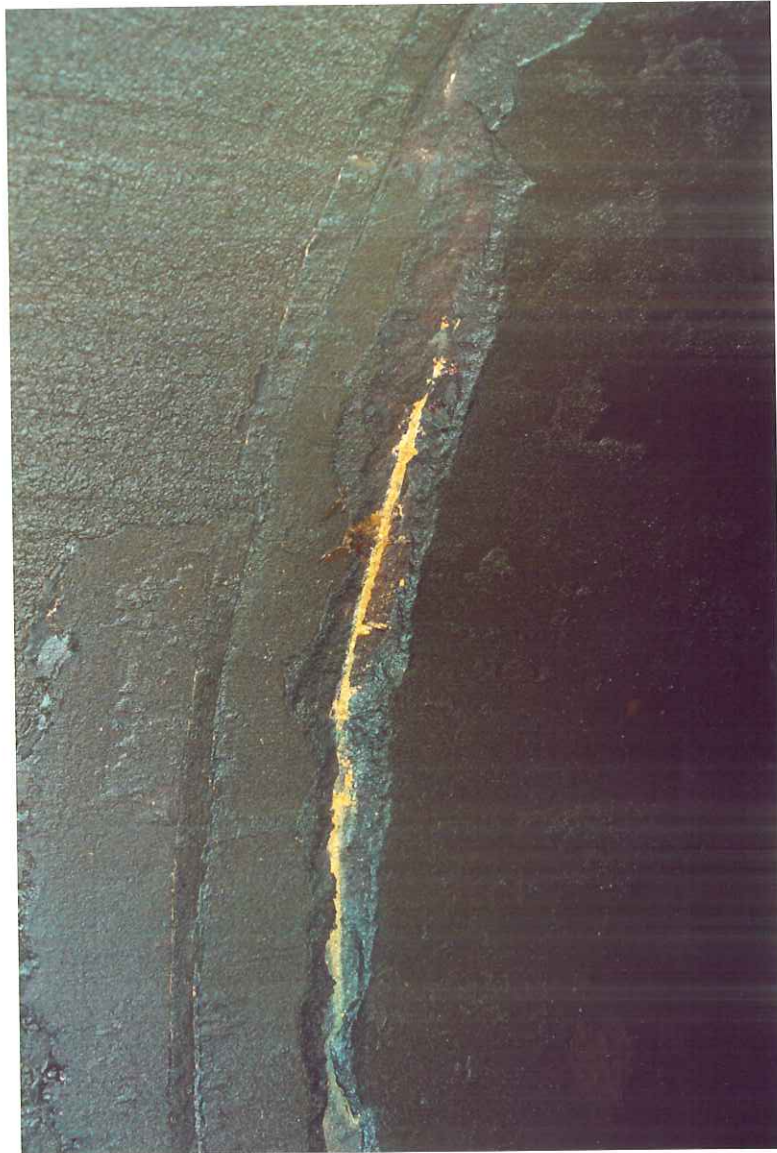
Figure 12. Spalled joint mortar and lining patch at the east springline at the north joint of the steel special with entry port at K2+952.
